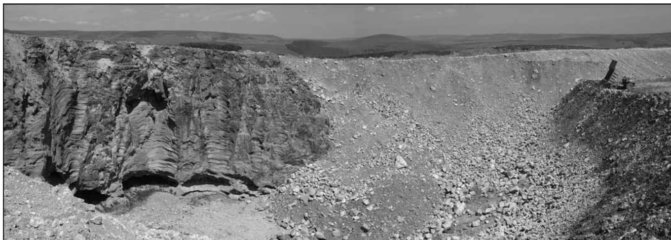
Backfilling the open pit in summer 2007. The tipper is on the fill at its intended level, which will finally reach a slope down to the foot of the face with the solution features.
